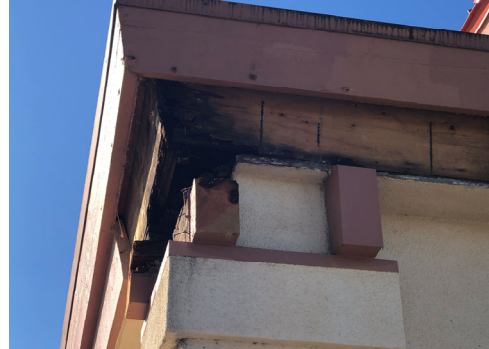
Additional dry-rot discovered that will need to be addressed in Phase 2.
