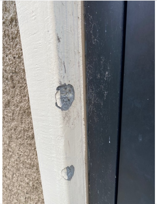
Damaged concrete trim
