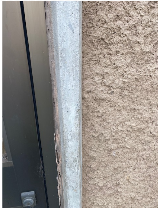
Damaged asbestos brown frame sealant-Building 1800A
