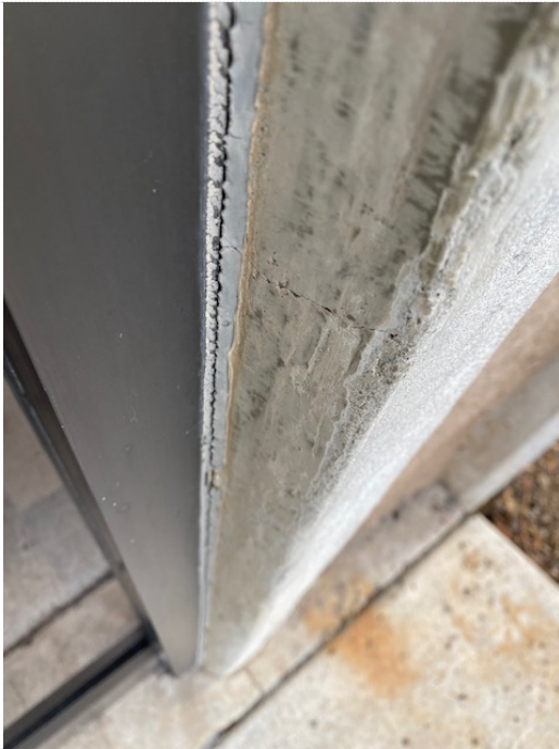
Damage to gray window sealant
