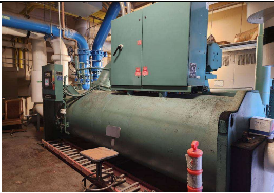
Existing Central Plant
