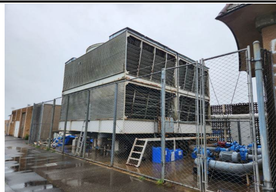
Existing Cooling Tower
