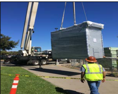
New equipment being delivered at Substation #1.
