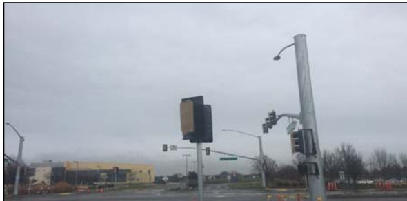
New Street Lights
