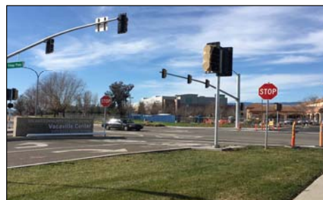
New Signal Poles
