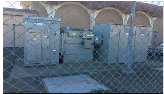
Substation #2 New Equipment
