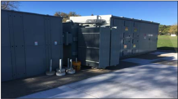
Substation #1 New Equipment
