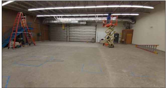
Robotics Lab Equipment Layout and Electrical Rough-In
