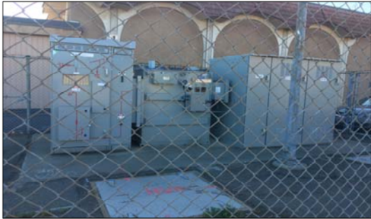
Substation #2 New Equipment
