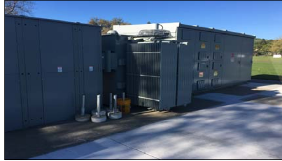
Substation #1 New Equipment
