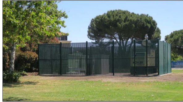
New B100 Generator Completed
