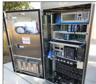
New Signal Lights Controller Cabinet
