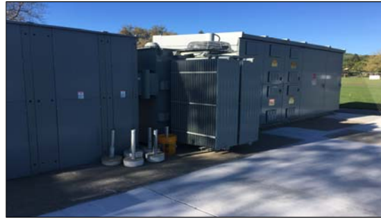
Substation #1 New Equipment
