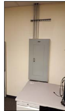
New HVAC Electrical Panel
