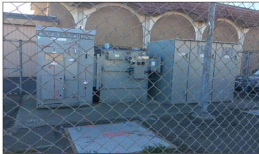
Substation #2 New Equipment
