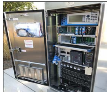
New Signal Lights Controller Cabinet
