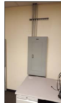
New HVAC Electrical Panel
