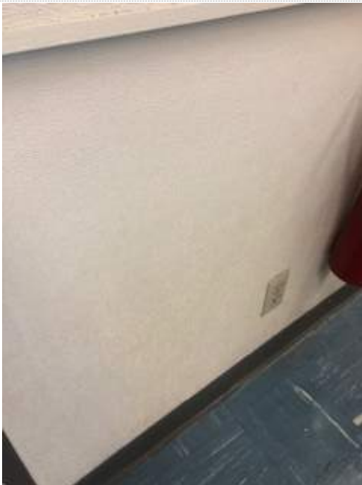
Sheetrock (<1% Chrysotile and 9" VFT with black Mastic (5% Chrysotile)
