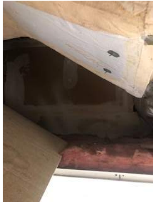
Duct Seam Tape-<1% Chrysotile
