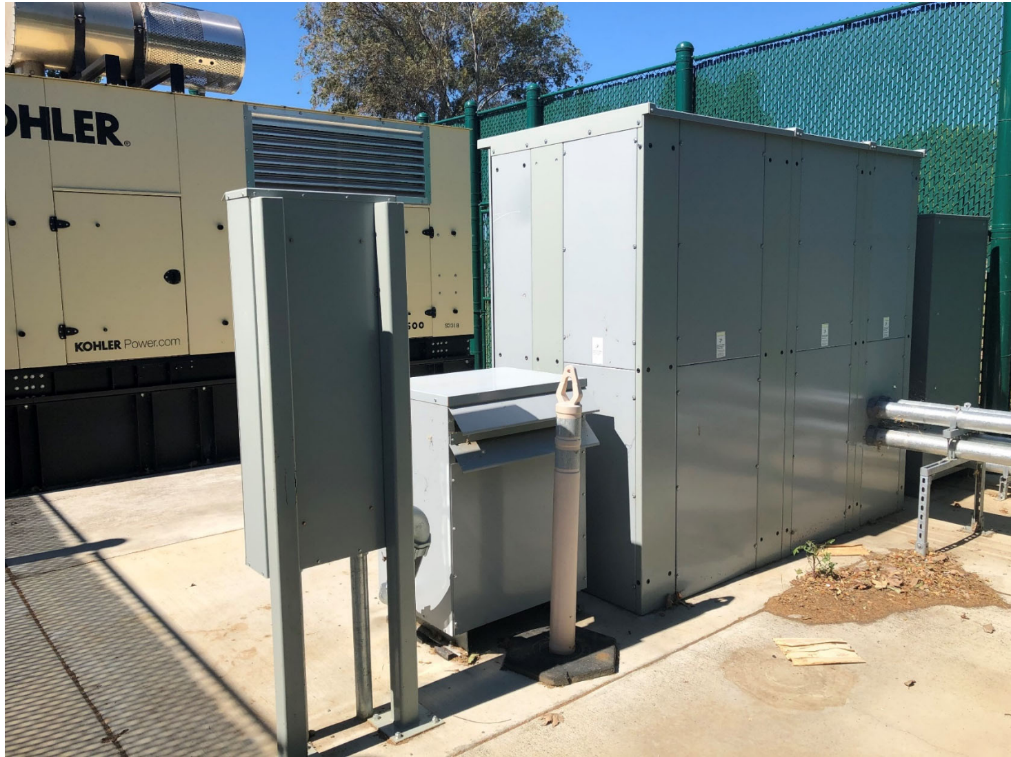
Substation #04 – Inside Fenced Area
