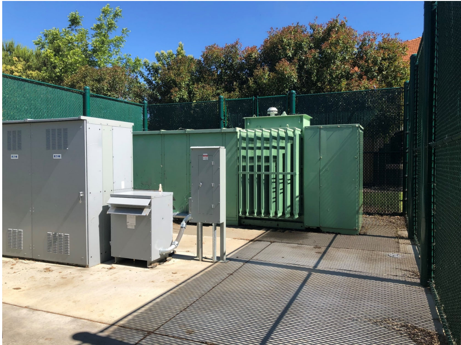
Substation #04 – Inside Fenced Area
