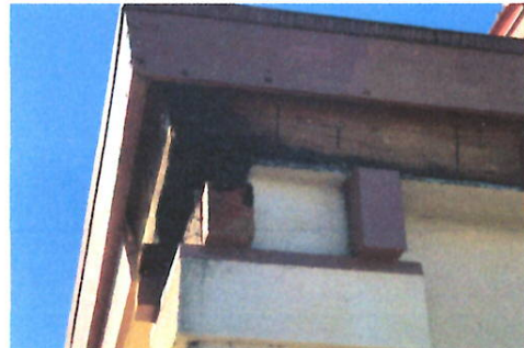
Additional dry-rot discovered that will need to be addressed in Phase 2.
