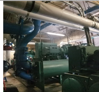
Existing Central Plant Photo
