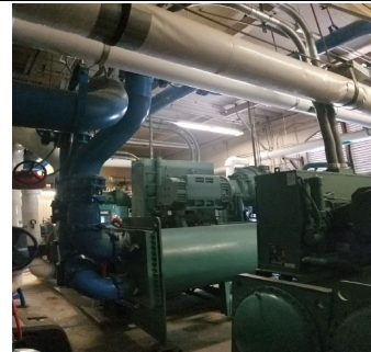
Existing Central Plant Photo
