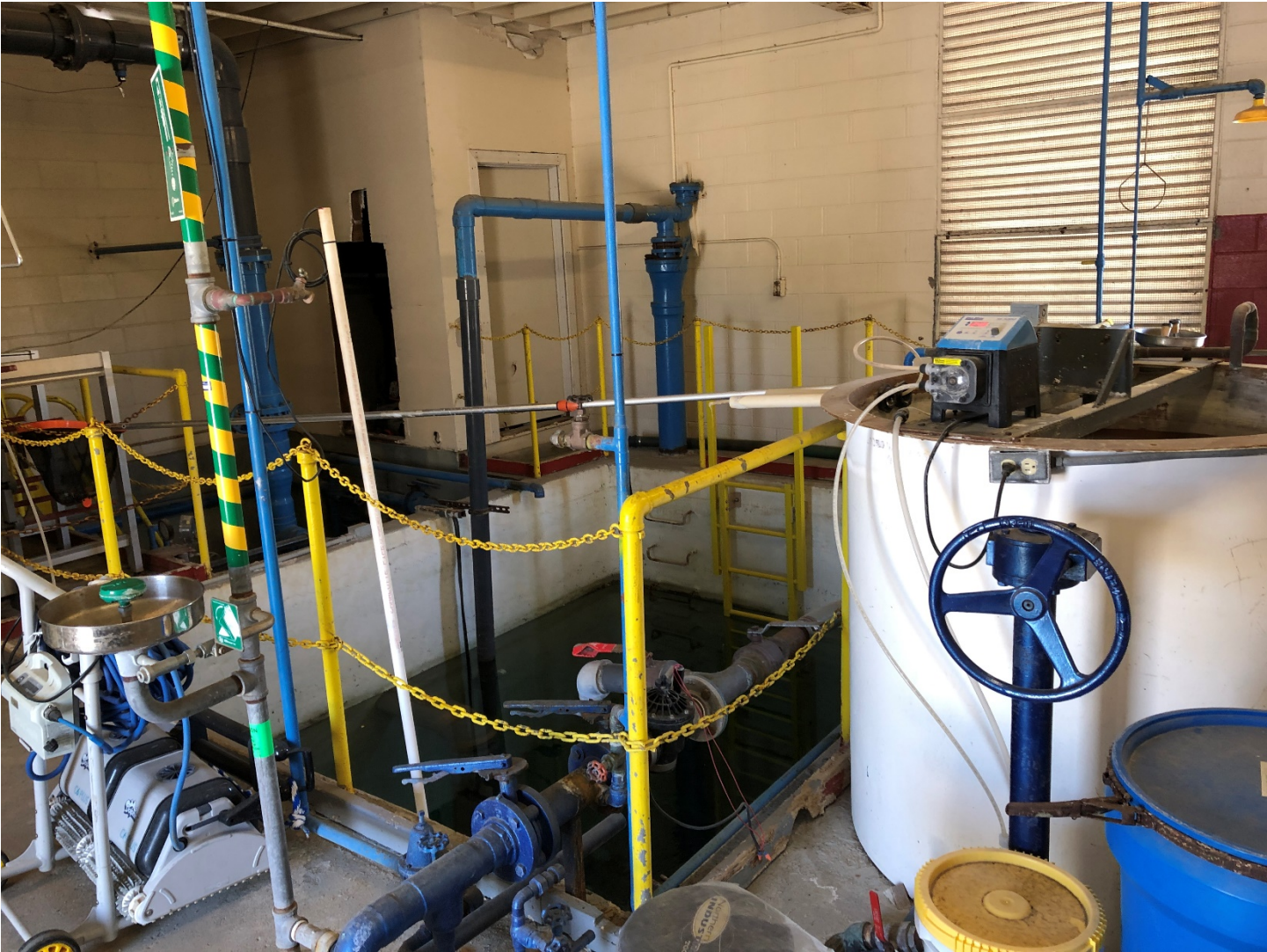
Pool Equipment Room (partial)
