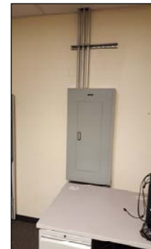
New HVAC Electrical Panel
