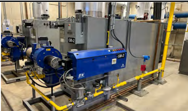
New Gas Boilers
