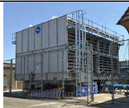
New Cooling Tower
